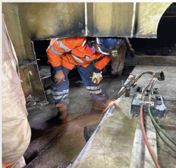
Cutting Damage Section
