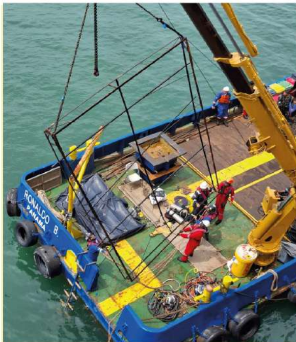
Divers taking templates of damaged sections
